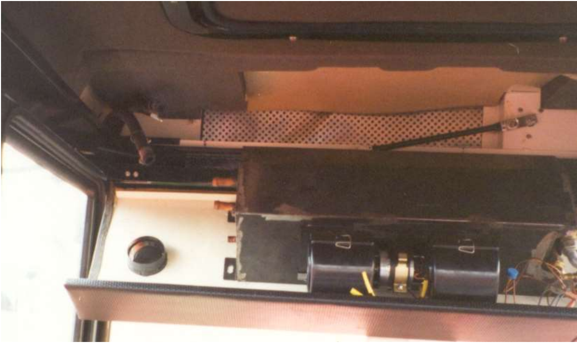
Heat/cool box showing heater side and necessary heater hose extensions.
